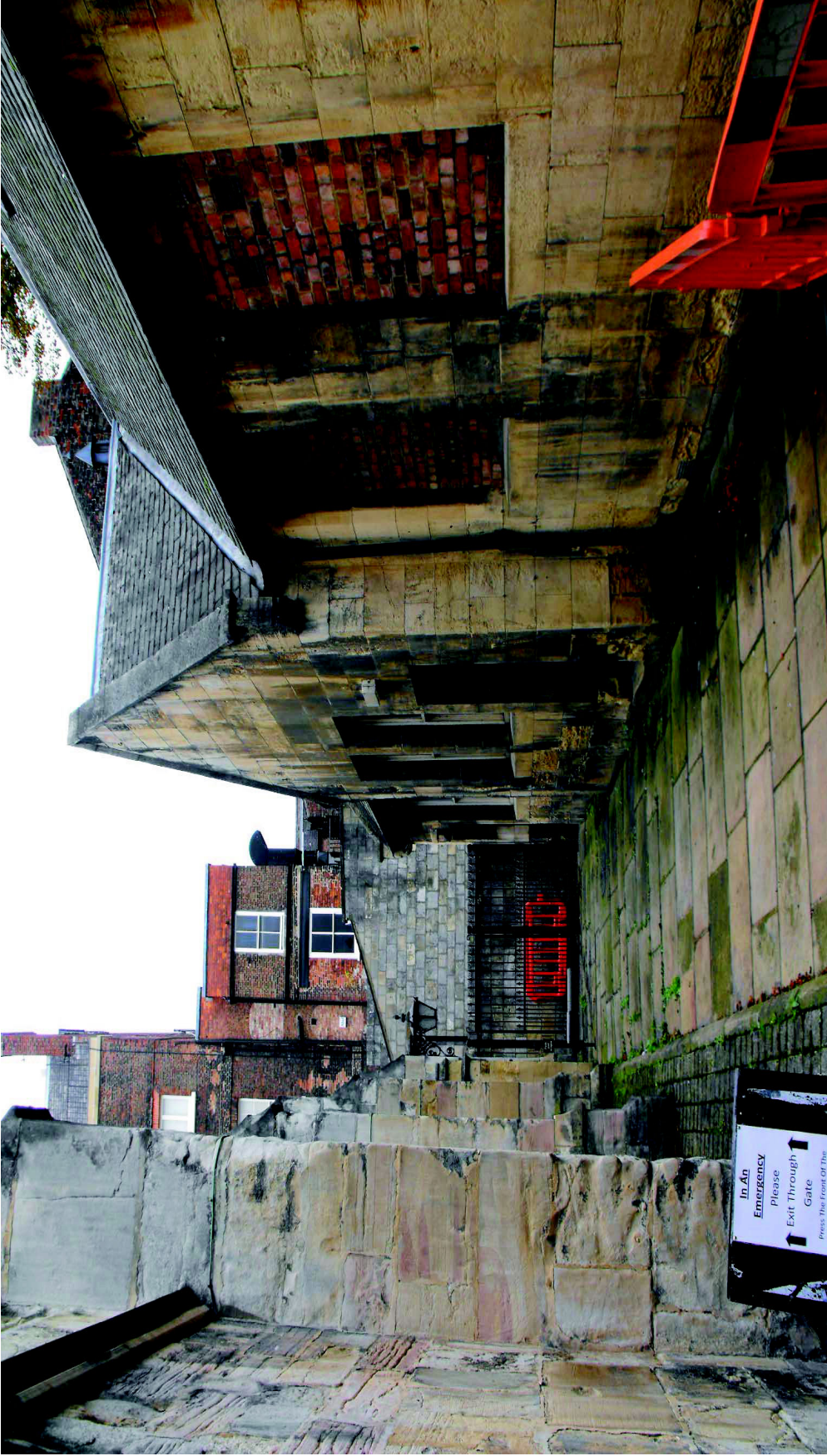
The East range and yard offer opportunity to form a glazed atrium space - providing separate access to toilets and meeting rooms from the Guildhall and Common Hall Yard.
