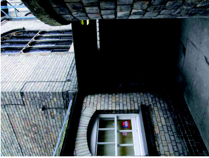
The existing Guildhall office entry is very unsatisfactory and not worthy of such an important Civic building. Accessibility is very poor.
